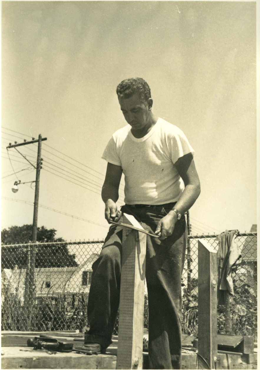
Carpenter working on beach stairs at the West End Racing Club - 1950's
