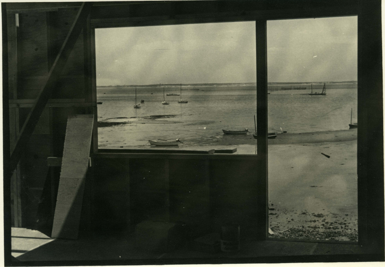
West End Racing Club under construction - 1950's View out the second story door and window Deck is not yet in place
